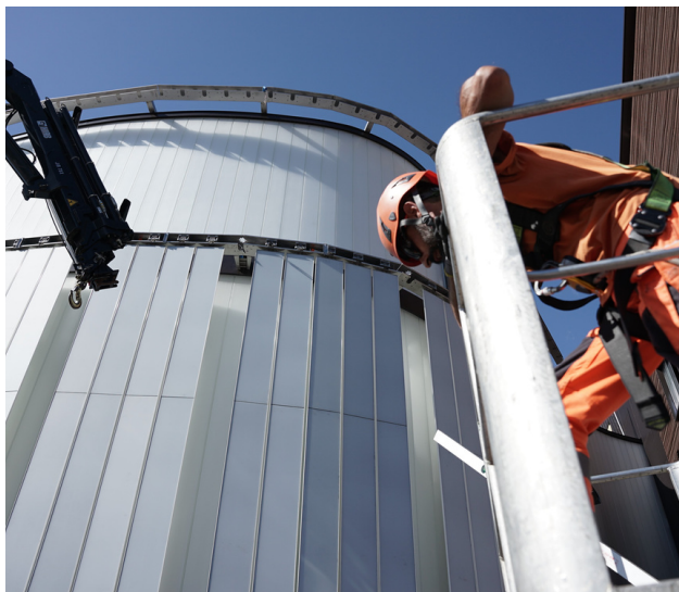
The BIPV system is installed on the new auditorium's facade on the complex's west side.
