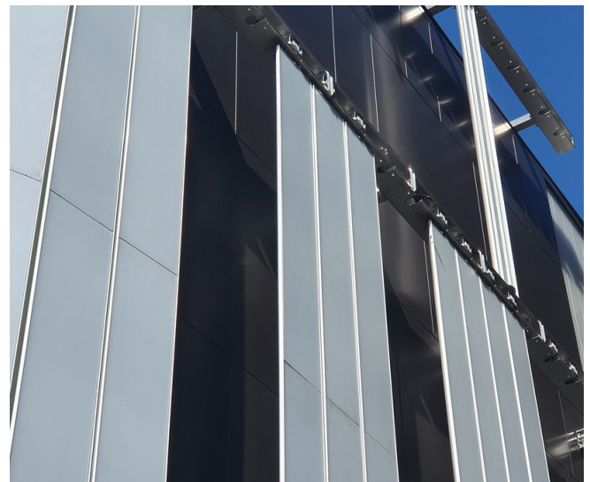
Close-up of the PV facade.
