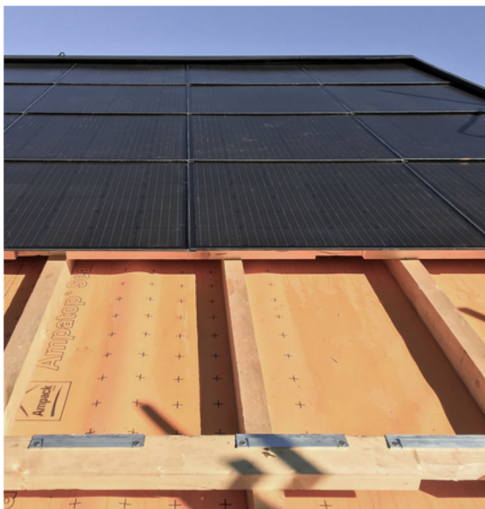
The photovoltaic modules are laid on top of the wooden roof battens.
