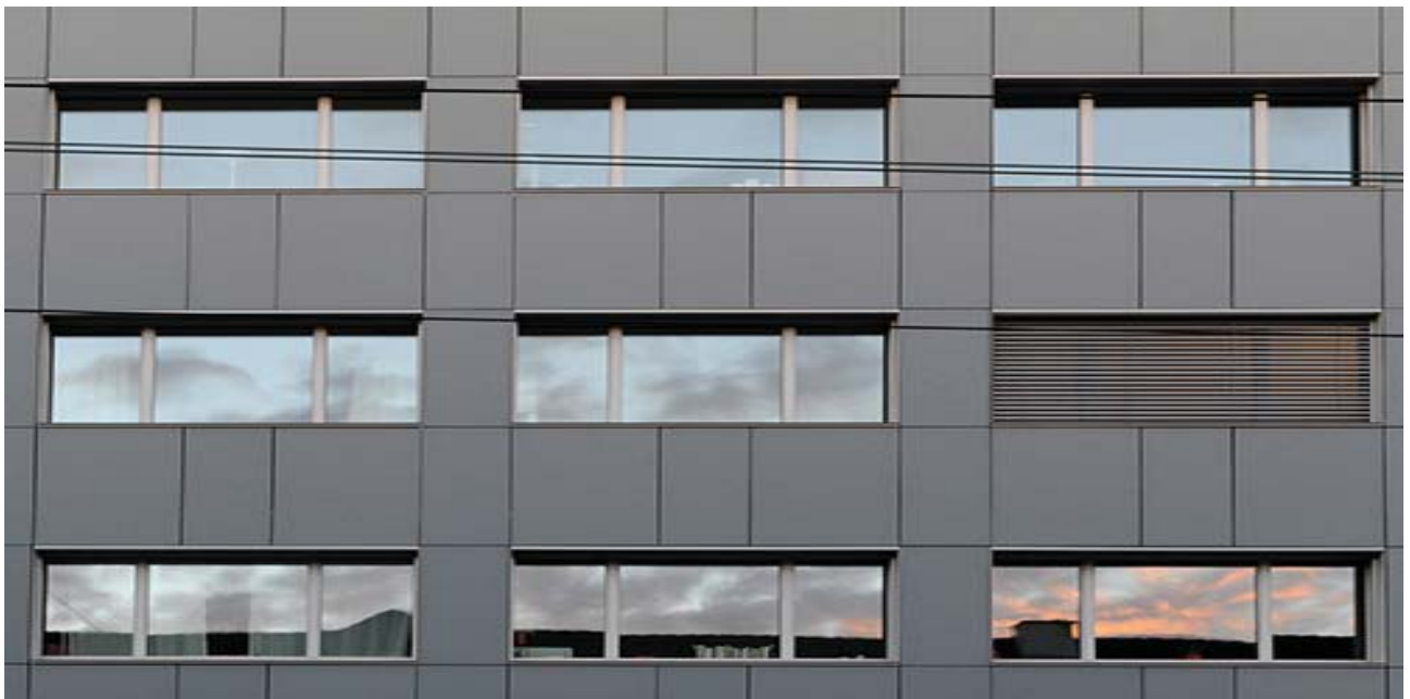
The realization of a BIPV facade requires the involvement of several actors at the same time.
