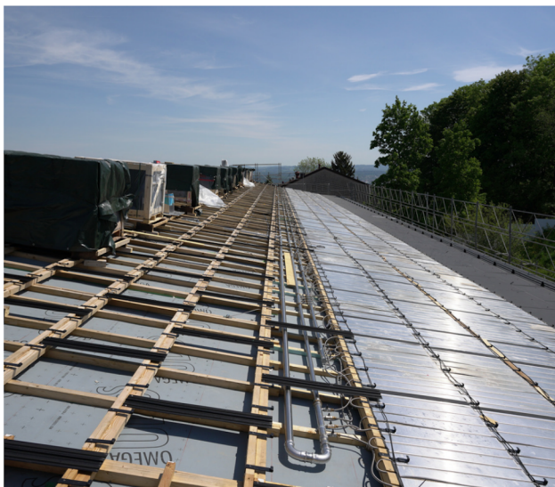
Photovoltaic tiles and PVT modules are integrated in the pitched roof.
